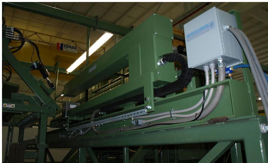
AGT800 Thickness Gauge installed on a 74" EPS Pickle Line
